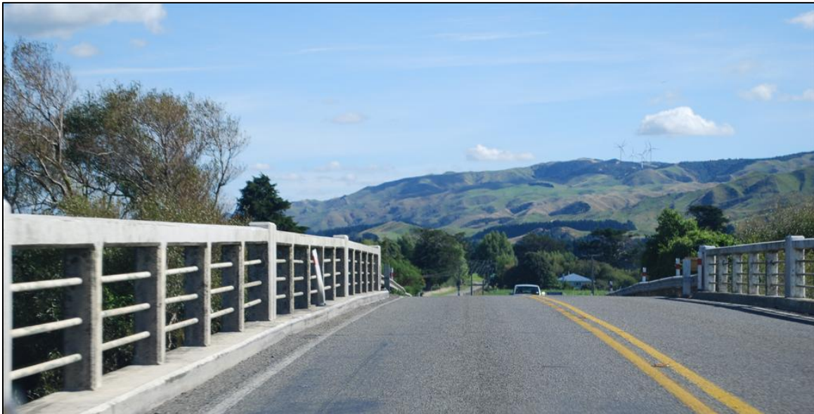
Figure 62: Many railway overbridges have inadequate shoulder width and may require clip-on bridges on each side for cycling safety (photo: Jonathan Kennett)
