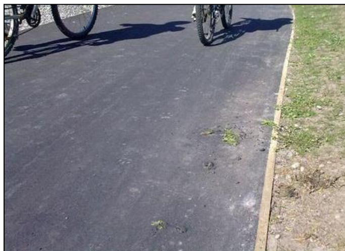
Figure 106: Vegetation growing through new asphaltic concrete path; good construction specifications and contract supervision are required
